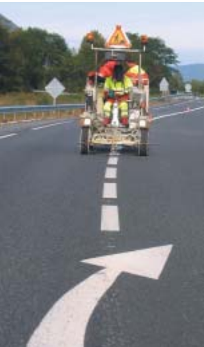
Upgrading road markings, a significant means of enhancing road safety at a reasonable price. Photo: Compagnie Signature, France
