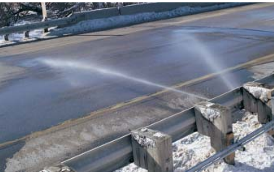
Safety on winter roads: anti-icing equipment installed in safety barriers. Photo: Quixote Transportation Systems, Inc., USA
